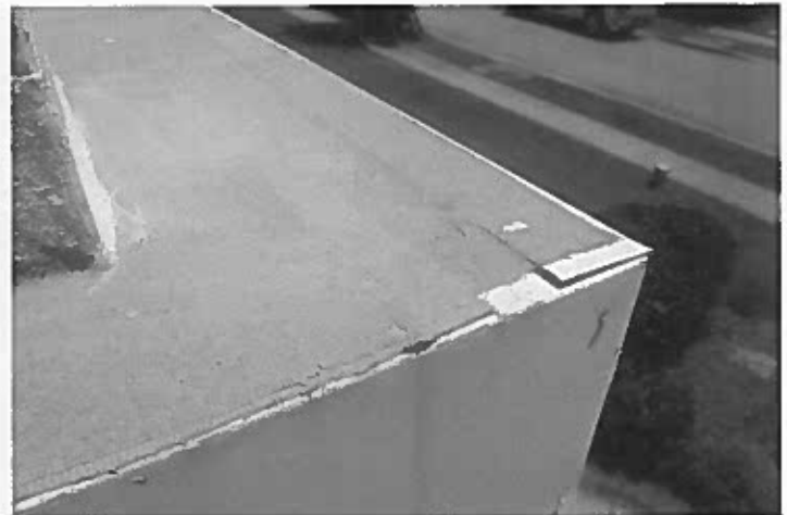
Figure 7. Component thickness prevents free drainage.
