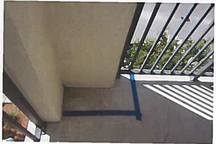
Figure 3. Integrated balcony column without drainage provisions.
